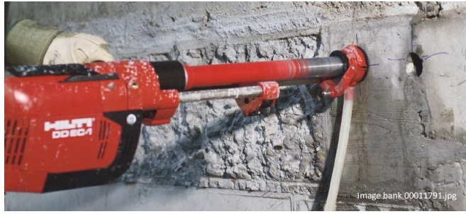
Figure 16 – Core drilling with a hand-held Hilti wet core drill with water-capture technology.
