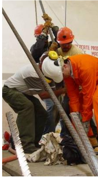
Figure 26 – Installing a long bar in an adhesive-filled hole can require the effort of several people
