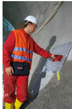
Figure 10 – Using a Hilti PS 200 hand-held ferroskan scanner to locate and map existing reinforcing prior to beginning drilling
